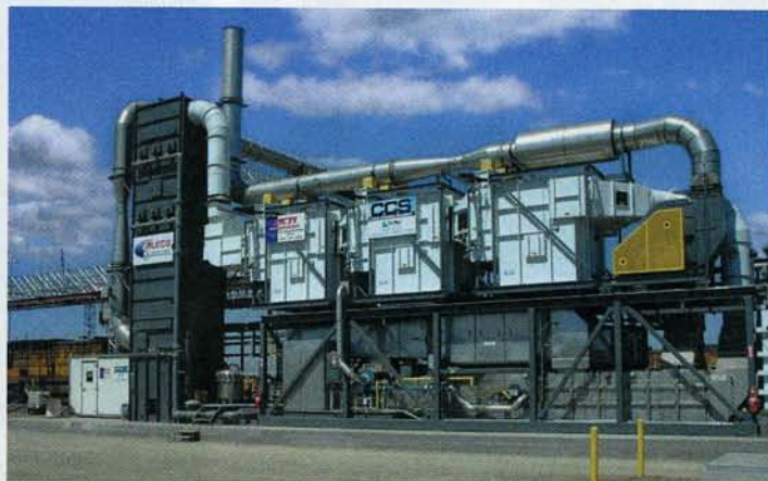
A Tri-Mer CCS gathers diesel emissions at the Union Pacific rail yard and Port of Long Beach.
